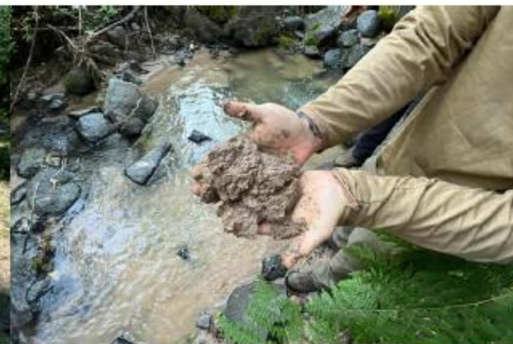
Lower Reach Road Erosion: Downstream Sediment at Culvert #1
