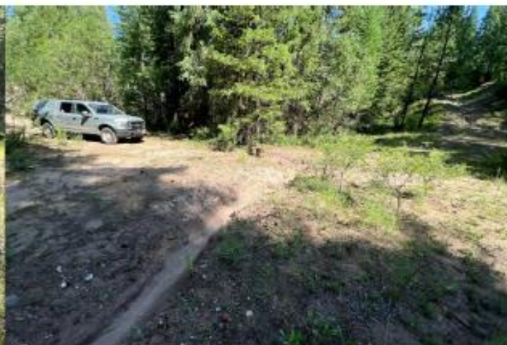
Lower Reach Road Erosion: Typical Road Damage & Headcut
