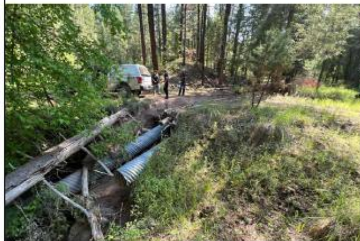
Lower Reach Road Erosion: Typical Culvert Damage & Headcut
